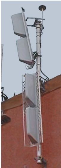
FIGURE 3: Telus Mobility 800-MHz paired grey analog and digital cellular site antennae with an attached GPS unit. (Image from Steve Rodaine's Cellular/PCS Antenna Identification Guide, www.geckobeach.com/cellular/cellpixs/cellid.htm .)
